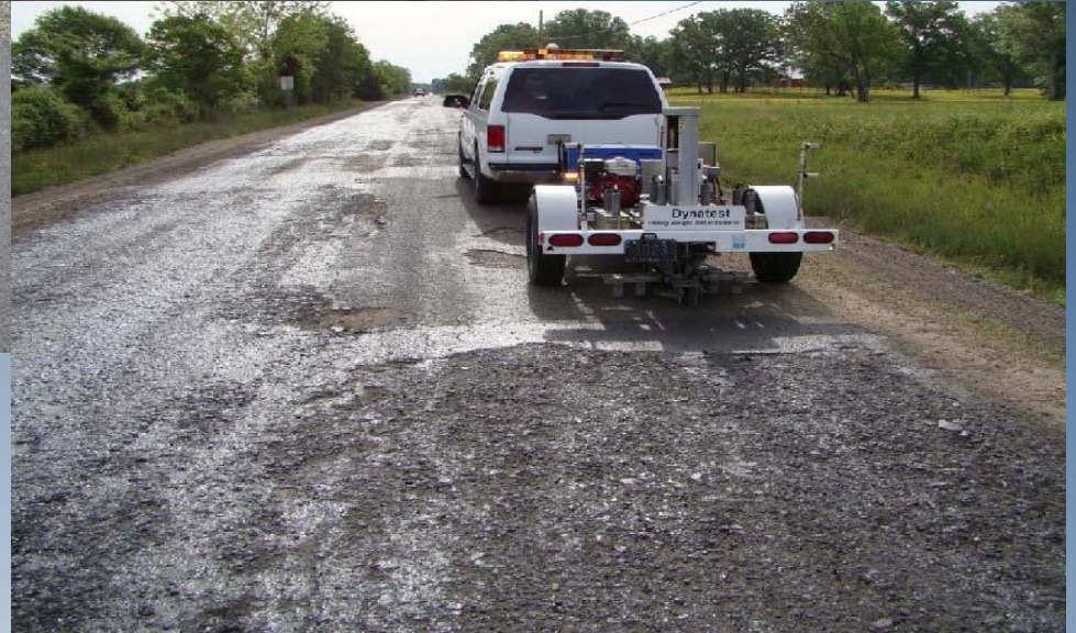
Total Asphalt Erosion
